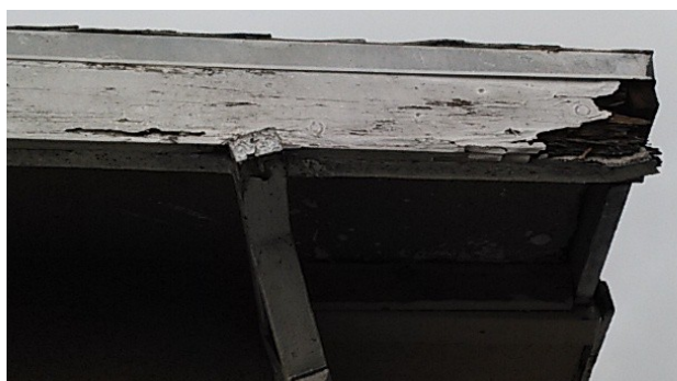
Figure 4: Termite damage, before “repairs.”
