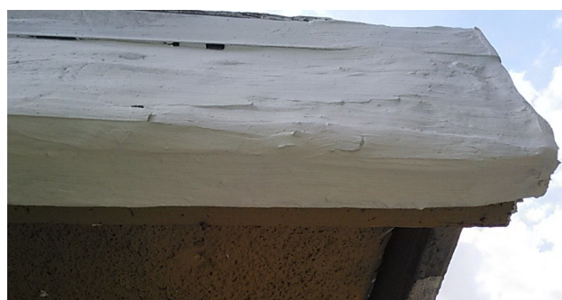
Figure 5: Voila! “Repairs” made. White goop spread over rotten wood. Very much SOP around these parts. (Update: 6-8-23. Further repairs made since then).
