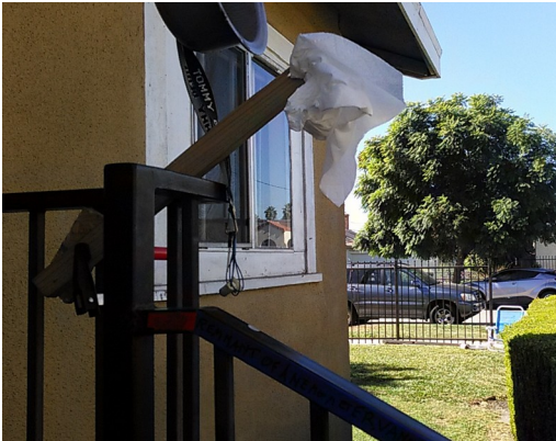
Figure 11: The broken base of the above-mentioned anemometer mast. To the right, the upper part of this ==> same anemometer mast, lying on its side behind bushes along with the damaged wind cups formerly mounted on top
