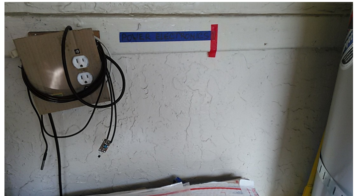
Figure 8: An electronic unit to control AC to a chest freezer converted to a fridge
